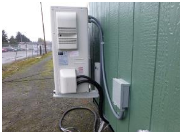
Figure 11. Location of disconnect box
