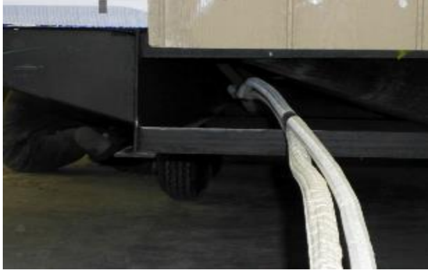
Figure 14. DHP refrigerant lines run along the chassis
