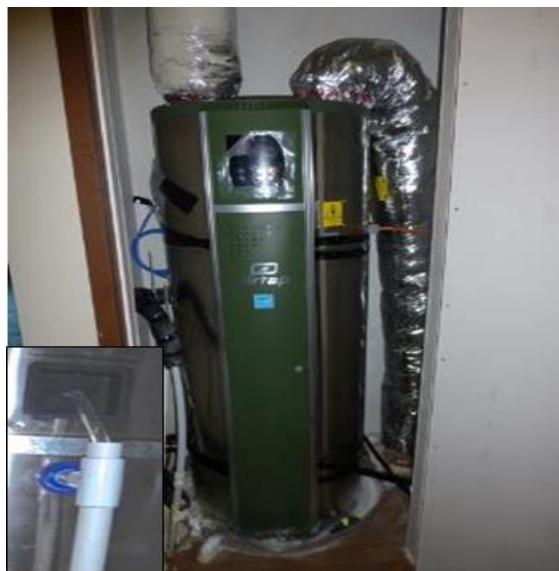
Figure 15. HPWH with ducting and condensate detail
