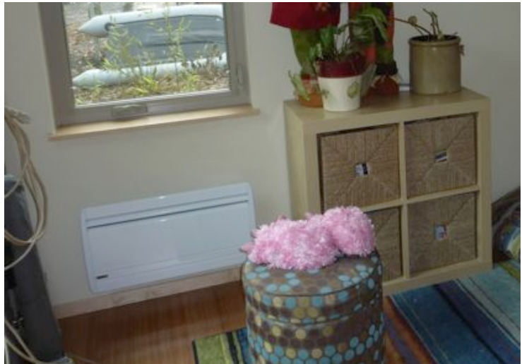
Figure 19. Electric resistance wall heater in bedroom
