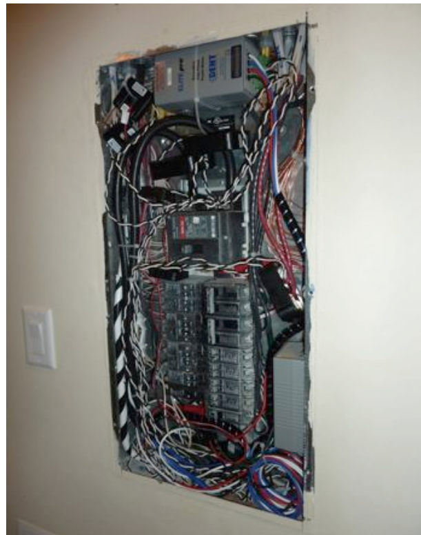
Figure 5. Data loggers inside main panel
