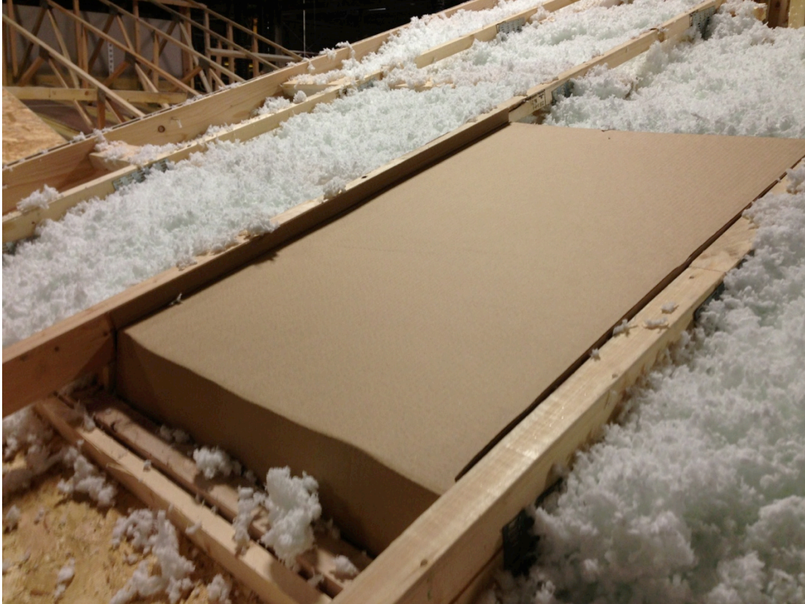
Figure 10. Baffle retaining compressed loose-fill insulation near eave
