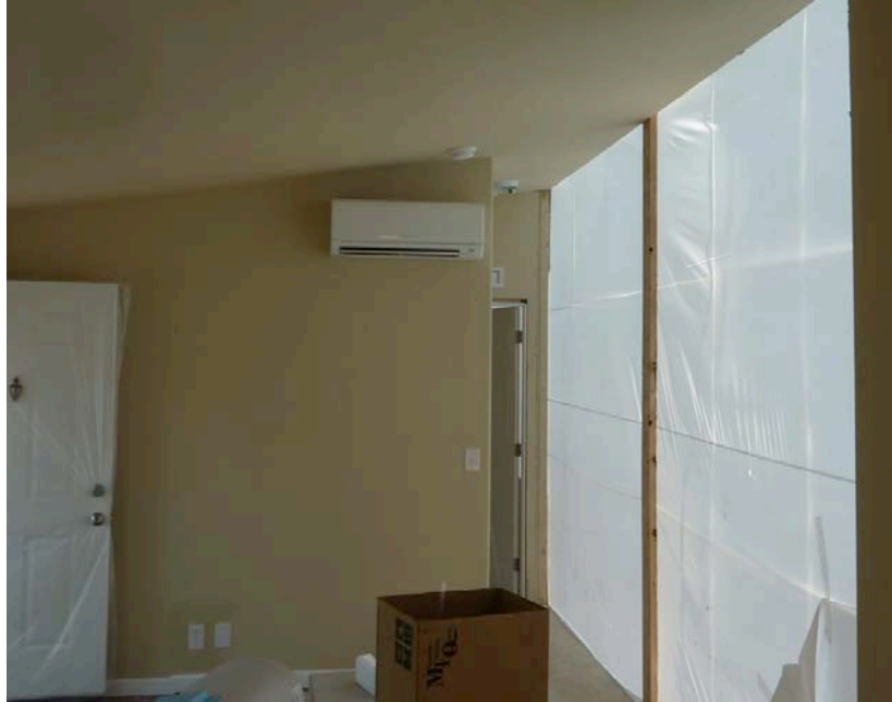
Figure 12. DHP indoor head mounted in main zone
