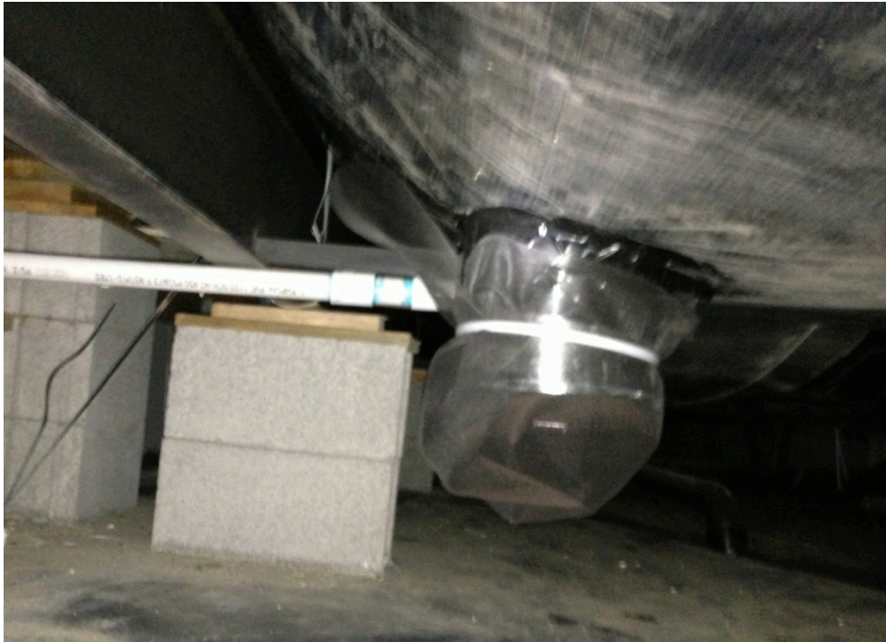
Figure 15. HPWH screened inlet located in vented crawlspace
